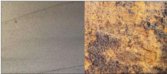
Fig. 3. Plate surface close-up. Left: intact plate. Right: c24 plate corroded and cleaned from corrosion products
