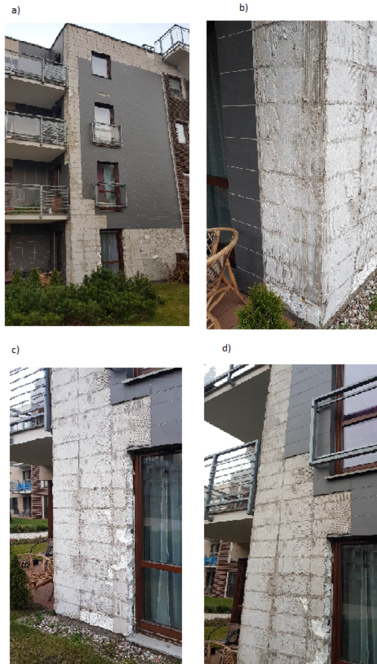
Figure 1. Damaged ceramic cladding a), b), c) and d) of the building facade
