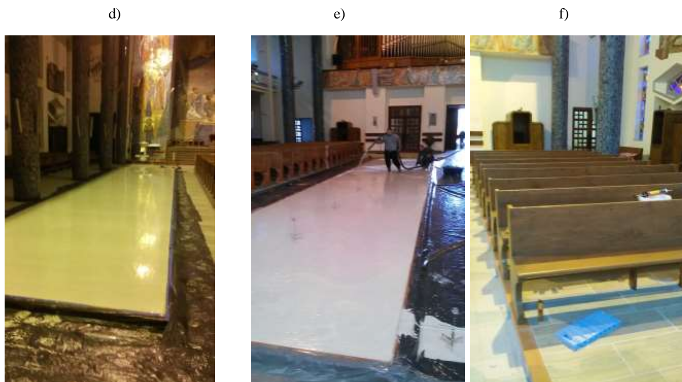
Photo 19: Installation of underfloor heating in the Church of the SHoJ in Gdynia in the rooms of the so-called of the upper church: a), b), c), d), e), f) stages of work (photo by Jacek Bramorski)
