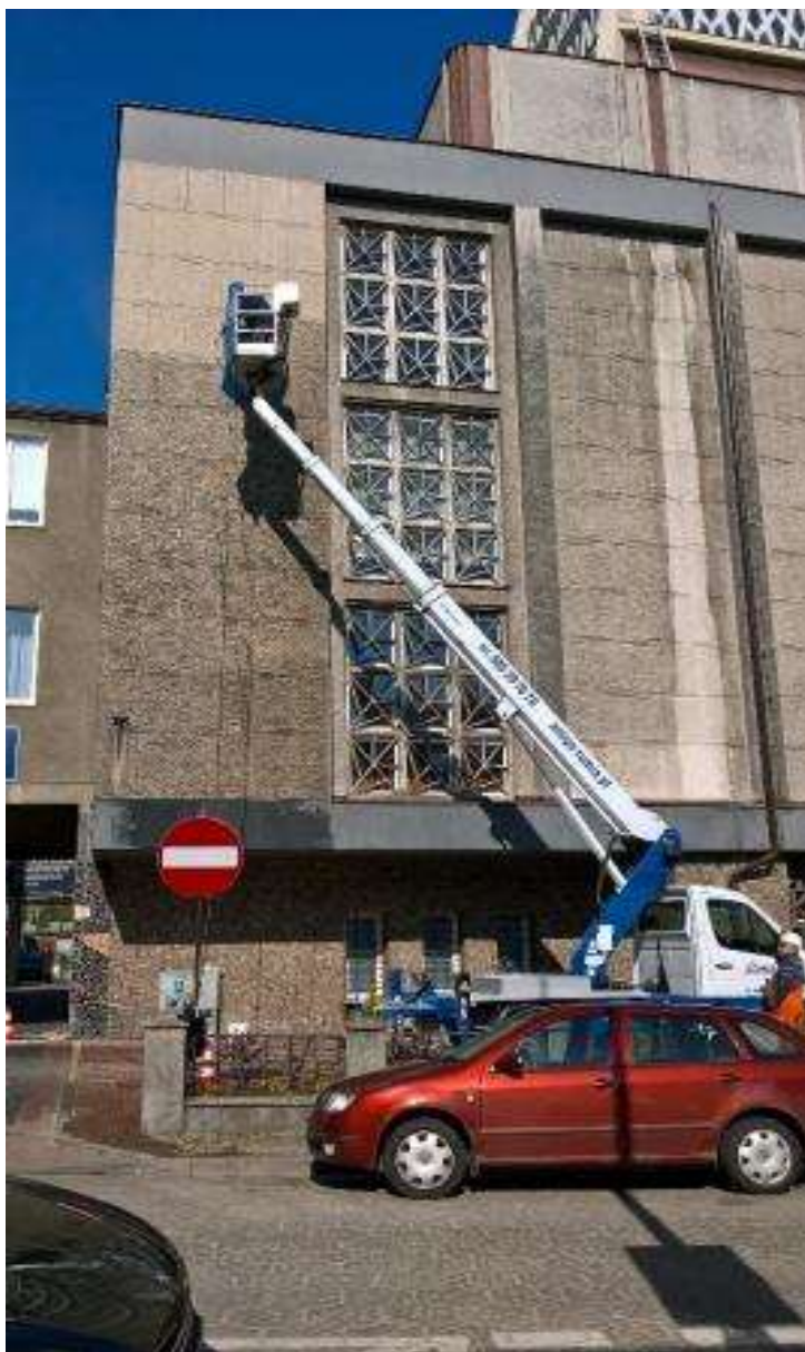
Photo 17. Comparison of the structure and color of the facade a) before and b) after its cleaning - on the example of the eastern facade (from the side of Monsignore Hilarego Jastaka Street) (street names as of 2023) (photo by Jacek Bramorski)
