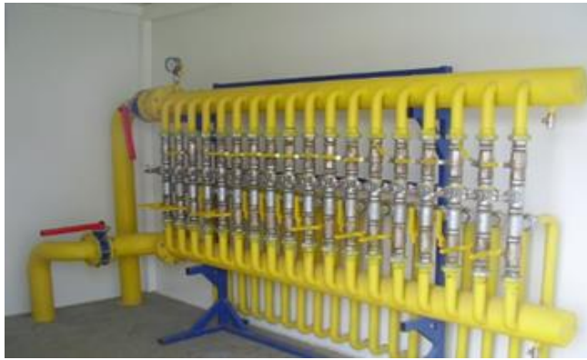
Fig. 3. Connection of gas wells to main pipelines (13)
