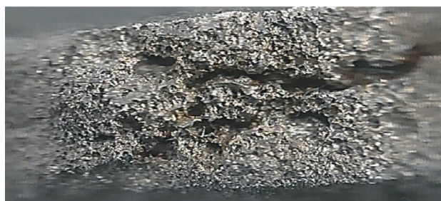
Fig. 1 Image of the corrosion coupon surface after exposition in the aqueous environment with H 2 S
