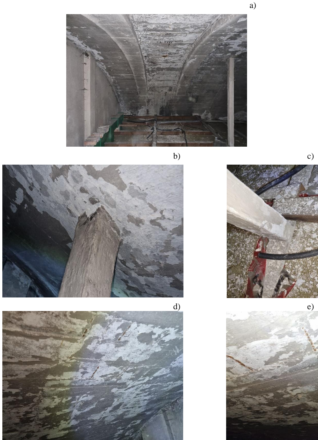
Photo 6. Warehouse building - attic space: a) stiffening ribs below the curvilinear covering slab, connection: b) post - curvilinear covering slab, c) post - horizontal tie, d), e) damage to the concrete cover of the reinforcing bars of the curvilinear covering slab
