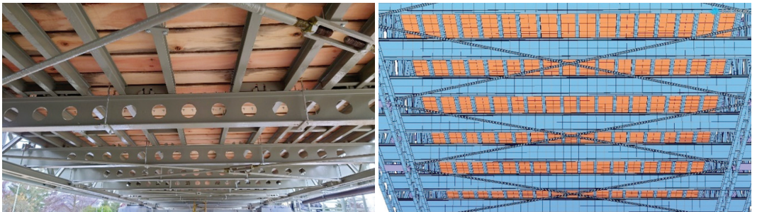
Figure 20. Bridge detail compared with the FEM model – bottom view on transoms, bracings, stringers, and platform deck
