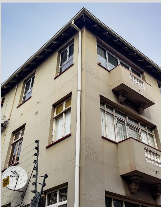
Figure 5-66 - Penmare (43 J.B. Marks Rd.) The original timber window frame (in poor condition) with coloured fanlight glazing is still contained on the 1 st floor, while the corresponding ground floor and 2 nd floor windows have been replaced. Unfortunately the 2 nd floor windows have not attempted to retain the frame colour or the casement proportions, a significant problem when replacing frames that affects the overall character.
