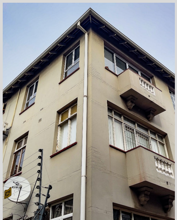
Figure 5-66 - Penmare (43 J.B. Marks Rd.) The original timber window frame (in poor condition) with coloured fanlight glazing is still contained on the 1 st floor, while the corresponding ground floor and 2 nd floor windows have been replaced. Unfortunately the 2 nd floor windows have not attempted to retain the frame colour or the casement proportions, a significant problem when replacing frames that affects the overall character.
