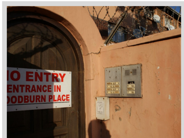
Figure 2-57 - Hennet Court, 1955, 328 Che Guevara Rd. The lack of maintenance, subsequent installation of visually intimidating security measures such as the barbed wire that is rusting, and the reduction of street surveillance through the construction of a solid boundary wall leads to a compromised image of a sense of security on the street.
