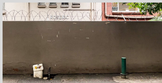
Figure 5-23- Roseric (67 Lena Ahrens Rd.) The rather uncoordinated and considered addition of servicing elements. To the left is a water meter in a ‘tamper proof’ housing that has evidently been tampered with. To the right is a stub column for telephonic infrastructure. As can be seen by the pavement repairs, these are treated in an ad-hoc manner.
