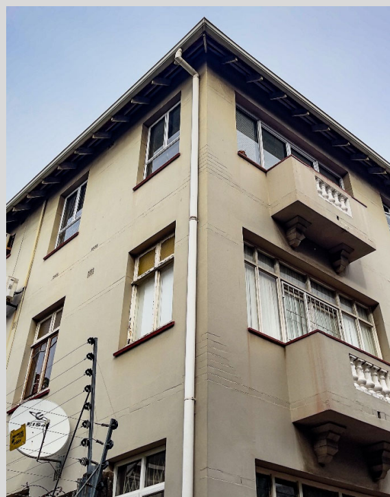
Figure 5-66 - Penmare (43 J.B. Marks Rd.) The original timber window frame (in poor condition) with coloured fanlight glazing is still contained on the 1 st floor, while the corresponding ground floor and 2 nd floor windows have been replaced. Unfortunately the 2 nd floor windows have not attempted to retain the frame colour or the casement proportions, a significant problem when replacing frames that affects the overall character.
