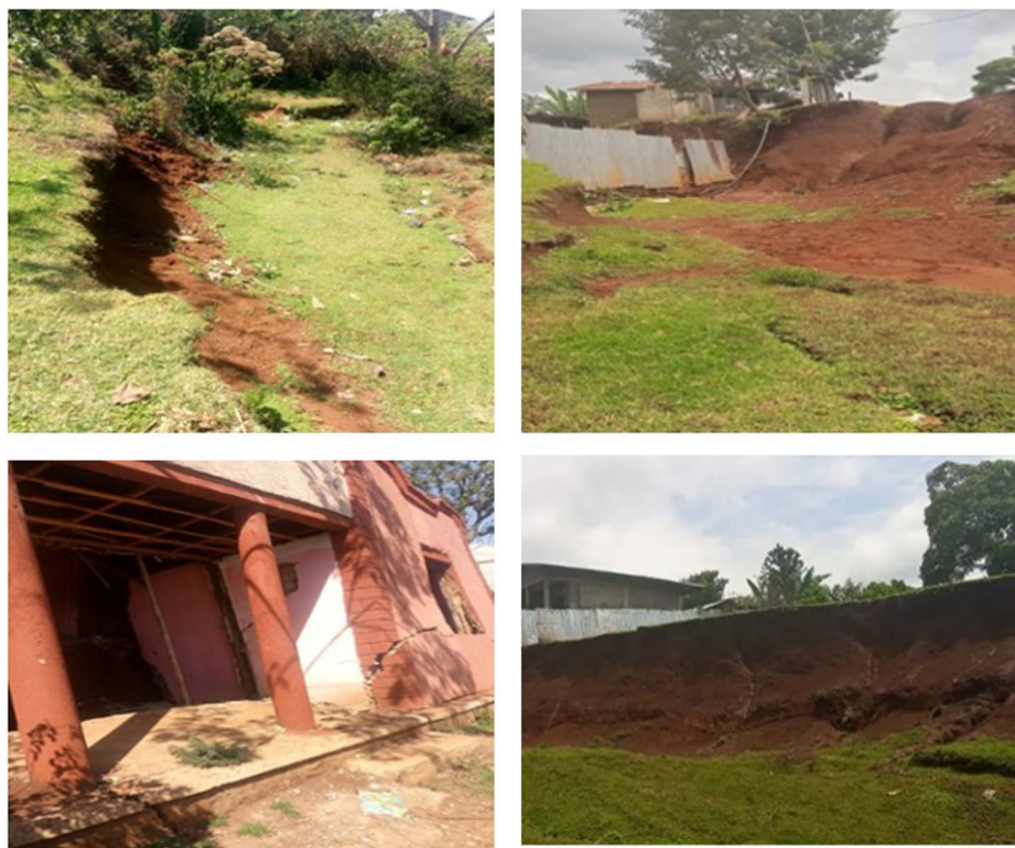
Figure 3. Land subsidence and effects on residential houses and roads.
