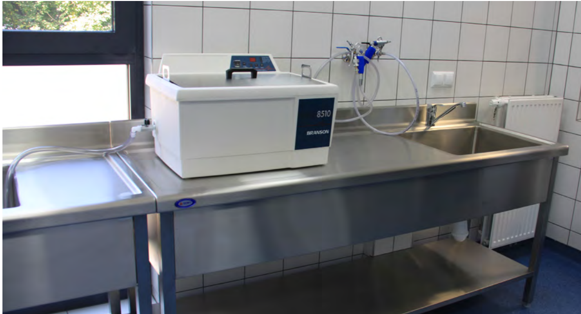
Photograph 2.1.2 A sterilisation unit (proper preparation of materials for sterilisation requires a number of activities to be performed); photographed by the Author, 2016
