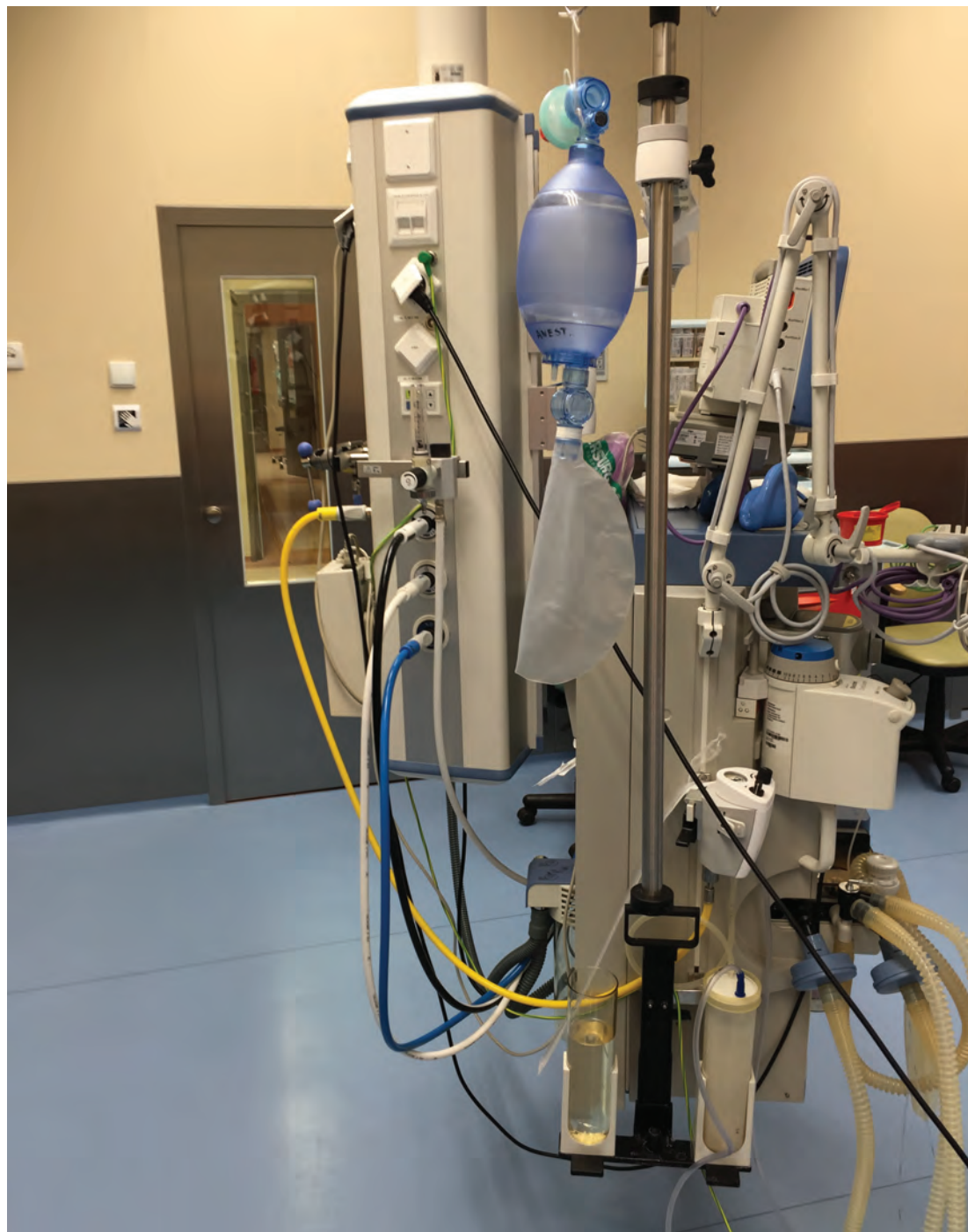
Photograph 6.2.3.6 The equipment in an operating theatre (a possibility of suspending some elements on a column facilitates disinfection of the floor); photographed by the Author, 2016
