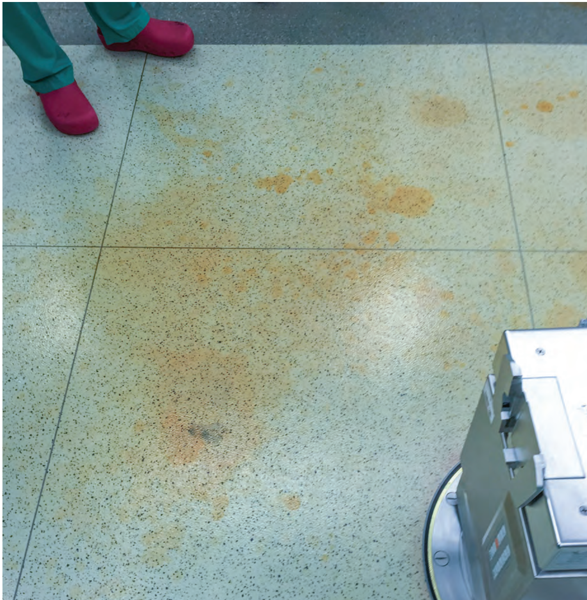
Photograph 6.5.4 A fragment of floor covering next to an operating table damaged by disinfectant agents (finishing materials should be adjusted to chemical agents applied during the procedures); photographed by the Author, 2016
