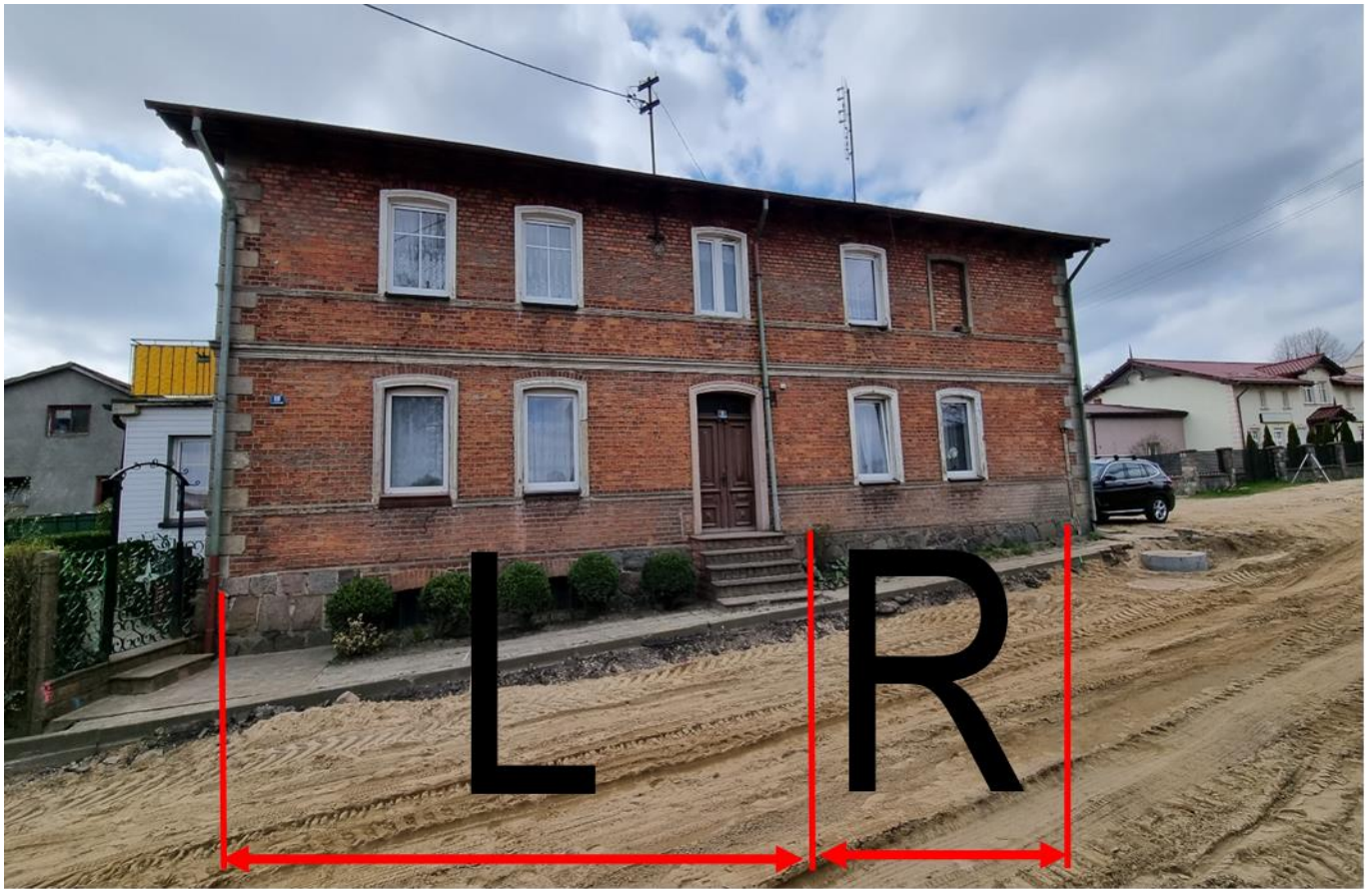
Fig. 1: Basement diagram of a residential building: (L): basement part, right side (R): part without basement, left side
