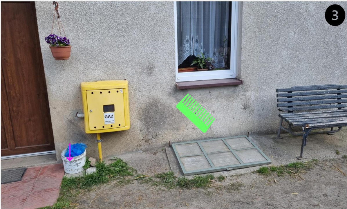
Fig. 6: Proposed location of target plates, benchmarks and feeler gauges on the external walls of a residential building: 1) front elevation (north), 2) side elevation (east), 3) garden elevation (south), 4) side elevation (west)
