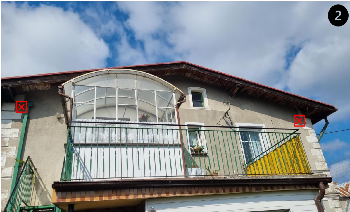
Fig. 6: Proposed location of target plates, benchmarks and feeler gauges on the external walls of a residential building: 1) front elevation (north), 2) side elevation (east), 3) garden elevation (south), 4) side elevation (west)
