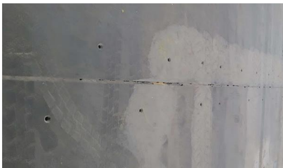
Fig.15. Concrete industrial floor (Example 4) during repair: diagram of drilled holes for injection feeding [38]
